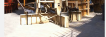
On the roof of the building, C&C installed a 40-foot (12m) lattice tower and cross-base by clamping it directly to the concrete floor it sat on.
